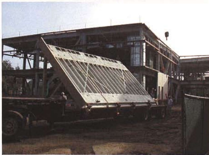
Because the thin-shell panels are lightweight, they could be fabricated in sizes up to 16 ft high by 40 ft long. Special handling procedures were required to transport the very large panels to the job site.
