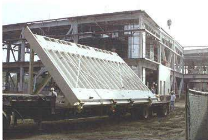
The large panels had to be shipped on a slanted easel at a 35-degree angle to be able to pass under a highway overpass. All panels traveled 80 miles without a crack.
